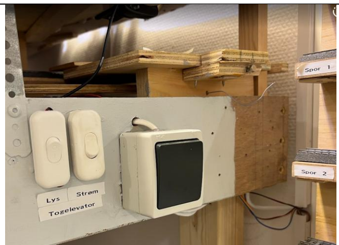
Manual switches for lights and power.
